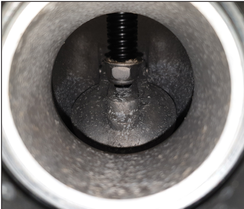
Screw down valve, view through the connector showing the spindle with the Nyloc nut and washer fitted to the end of the spindle.
